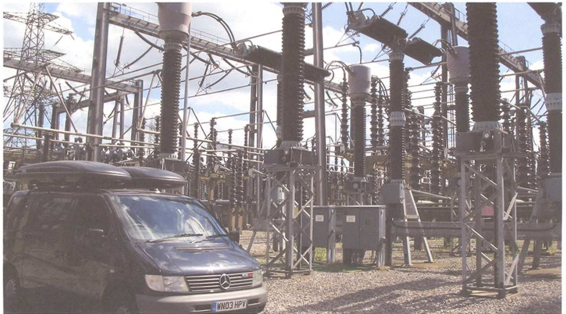
On guard: A new system developed at the University of Strathclyde 'listens' for tell-tale radio signals which give advance warning of potentially dangerous electricity sub-station faults.
